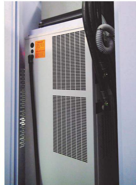
油霧回收器及冷卻系統 Mist collector and cooling system
